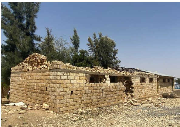
Classroom block looted during the conflict at Negash Primary School
